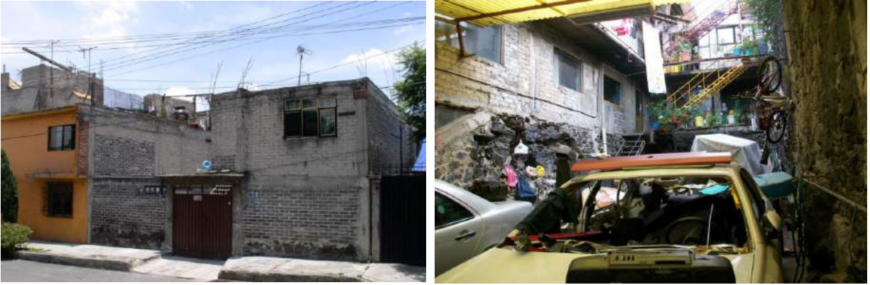
Photo 4.11. (left) Evidence of renting (4 electric meters). Photo 4.12 (right) Renting between four households plus owner (13 people in total) and precarious stairs to second and third floors
