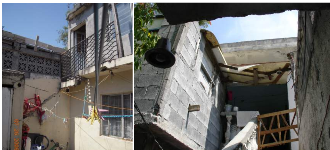
Photos 4.1 and 4.2. Dilapidation of homes in Monterrey.
