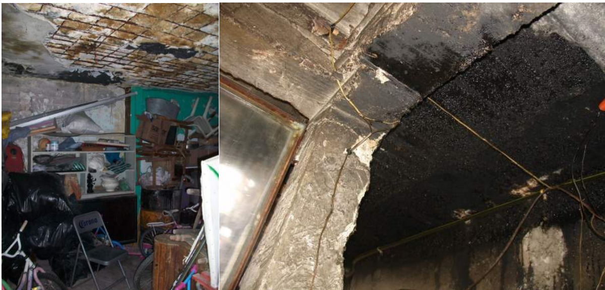
Photos 4.13 (left) and 4.14 (right). Hazardous conditions of leaking and collapsing roofs (left) and exposed wiring and evidence of fires caused by short circuits (right)
