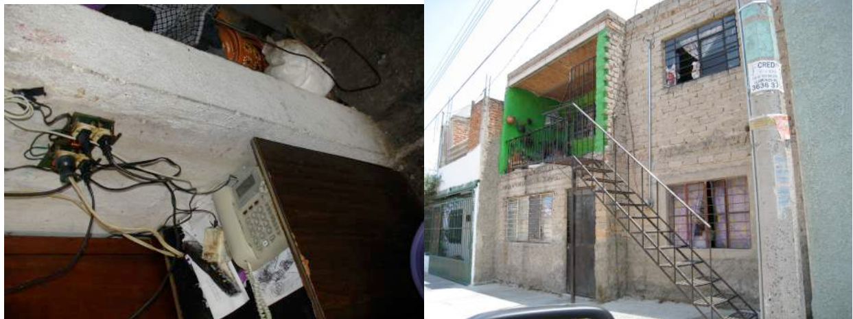
Photos 3.1 – 3.2. Self-production of the houses, problems with structure and installations: inadequate and overloaded electrical installations (left) and access to second floor dwelling from the sidewalk (right).
