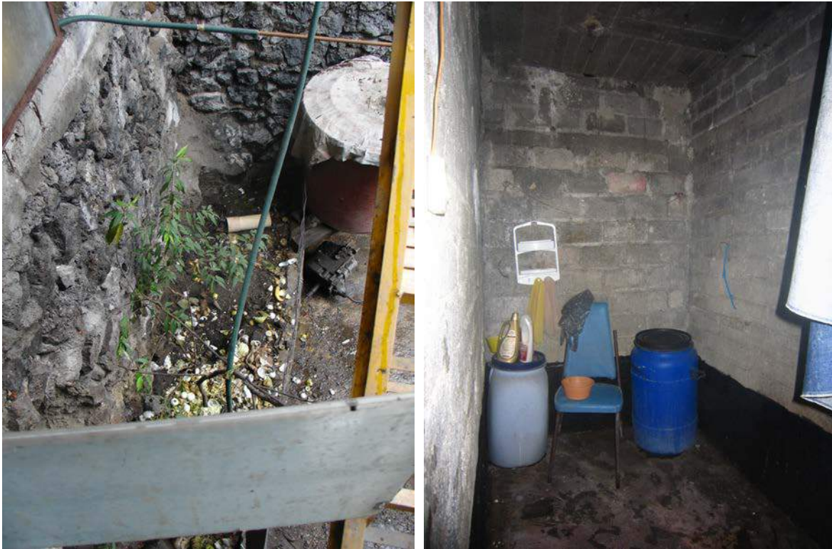
Photos 12.17 and 12.18. In Photo 12.17 (left) gas pipes (covered in green) cross over each other with a water tank below. The gas pipes are not attached to the wall. Each tenant makes his or her own installation and connection. Photo 12.18 (right) shows a common shower space. There is no actual shower; residents wash from buckets.
