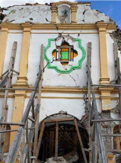
Photograph 3.2: Visible damage of the church in San Francisco Xochiteopan from the 2017 Earthquake (Image taken by Dr. Ricardo Ainslie in October 2019).
